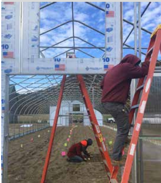
UMass now has a high tunnel we can conduct trials in! On October 26 th , before construction was complete and expecting a weekend of rain, The Vegetable Team seeded 15 varieties of spinach with downy mildew resistance. The tunnel is now skinned, and the spinach germinated. Stay tuned for results. Photo: K. Campbell-Nelson
